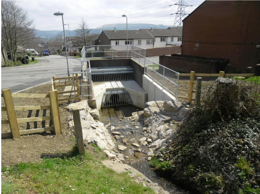
Image of one of the upgraded inlets built as part of the Rhydyfelin Flood Alleviation Scheme
