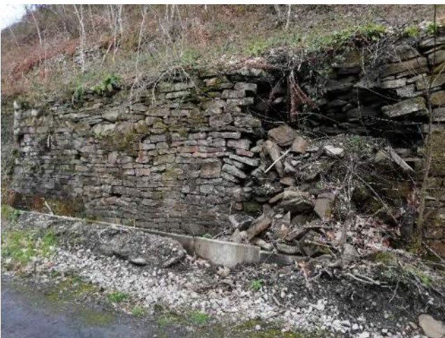
Figure 16 – wall in state of disrepair
