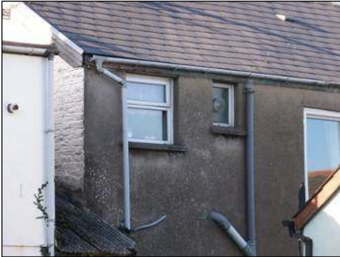
Loss of character through use of unsympathetic materials
