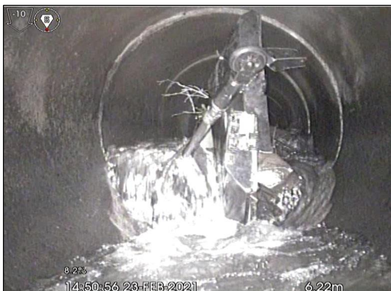
Figure 7: Obstruction identified approximately 6 meters downstream of the Swansea Road culvert inlet
