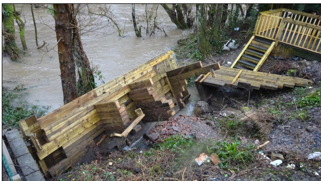
Figure 14: Damage to property caused by the River Cynon to the rear of Richmond Drive, Hirwaun on the 16 th February 2020 (image captured by resident)
