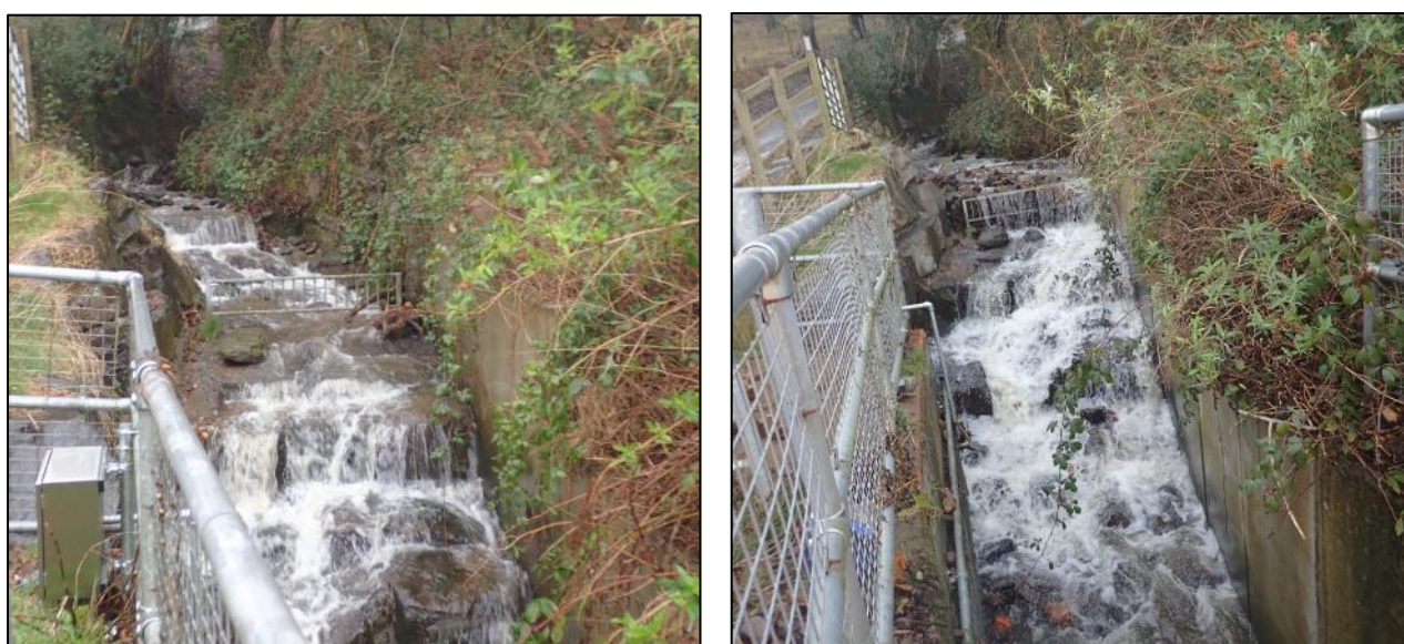
Figure 16: Upstream view of 'Culvert Inlet 1' before Storm Dennis (left) and post Storm Dennis (right) showing debris behind the upper debris screen (captured by RCT's Flood Risk Management team)
