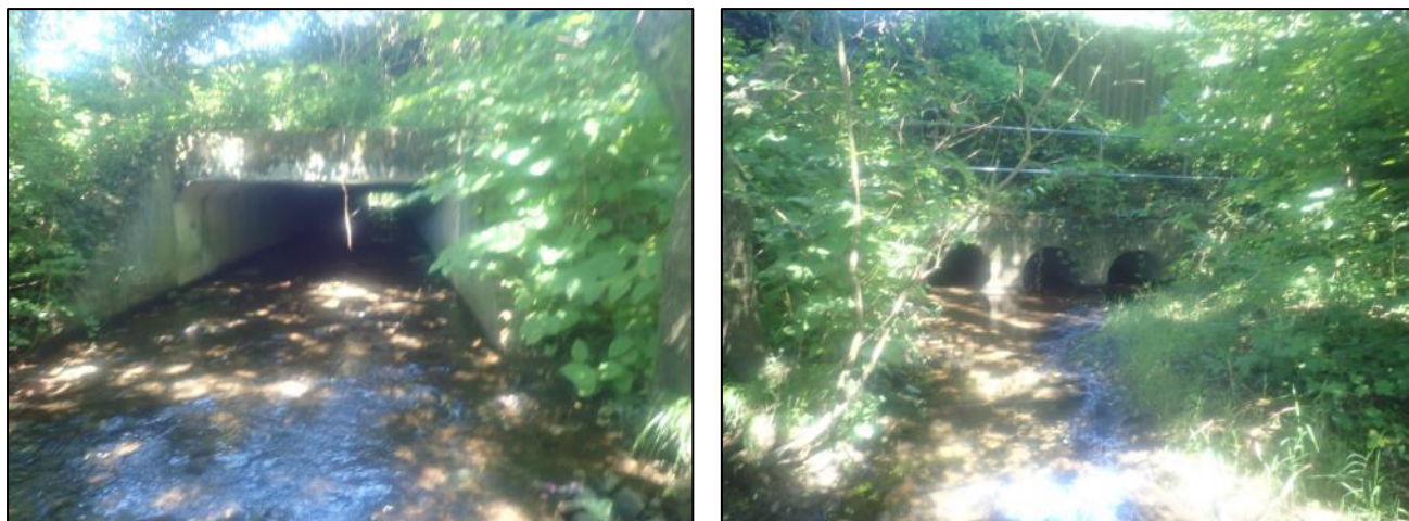
Figure 24: Nant Corrwg culvert outfall (left) and an unnamed ordinary watercourse culvert outfall (right) below the A470 (captured by RCT's Flood Risk Management team post event)
