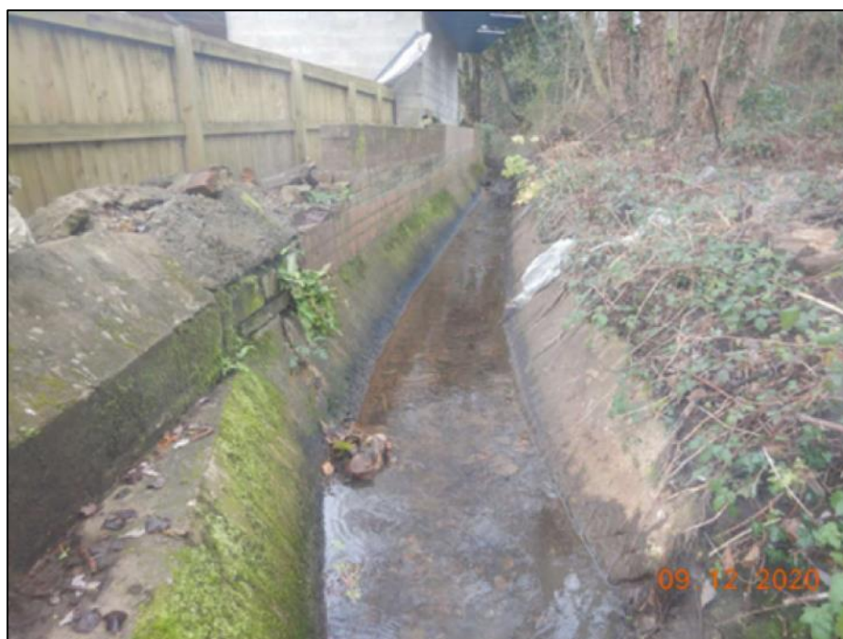
Figure 26: View of damaged channel retaining wall to the rear of Hawthorn Crescent looking upstream (captured by Edwards Diving Services post storm event)
