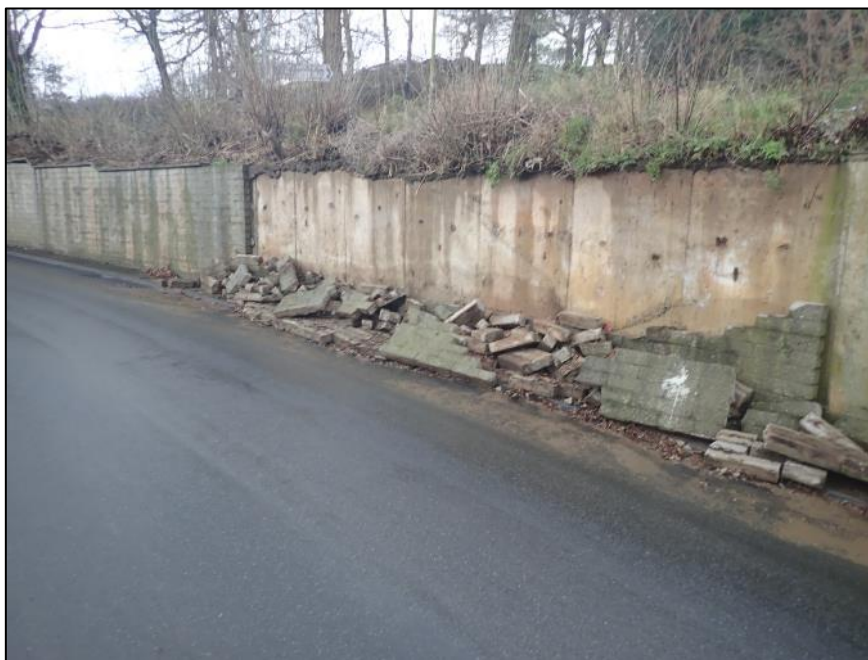
Figure 7: Damaged highway retaining wall below 'Culvert Inlet 1' (image captured by RCT's Flood Risk Management team on 17 th February 2020)
