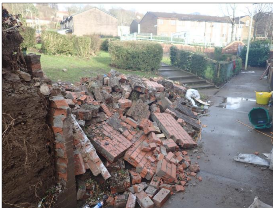
Figure 8: Damaged retaining wall at Wordsowrth Gardens caused by the surcharging of 'Culvert Inlet 1' (image captured by RCT's Flood Risk Management team on 17 th February 2020)
