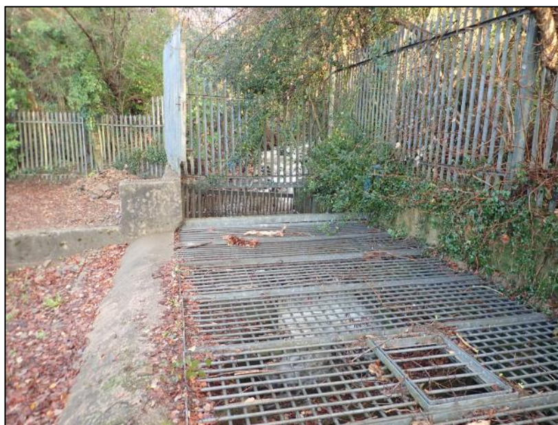
Figure 18: Image of 'Culvert Inlet 3' showing initial debris screen and safety grid (captured by RCT's Flood Risk Management team post event)
