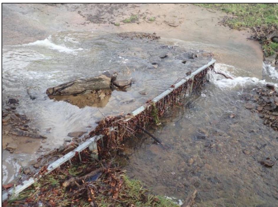
Figure 21: Evidence of debris trapped behind the upper debris screen above 'Culvert Inlet 2' (captured by RCT's Flood Risk Management team on 17 th February 2020)
