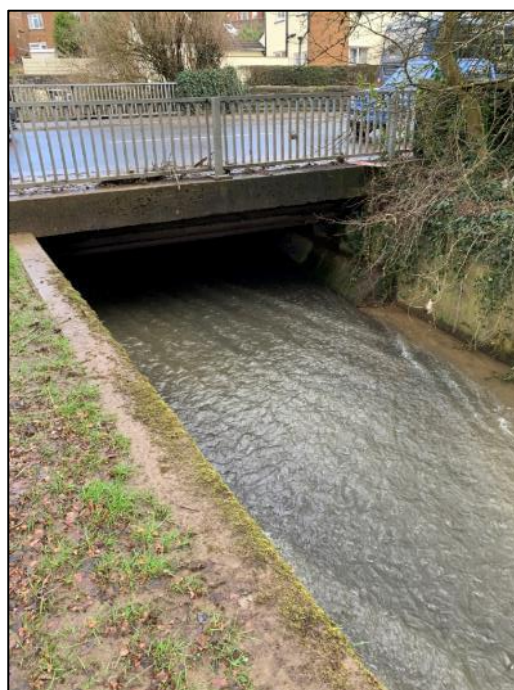
Figure 27: Nant Lonydd culvert outfall below the A4054 (Cardiff Road) which was identified as surcharging during Storm Dennis (image captured by RCT officers post event)
