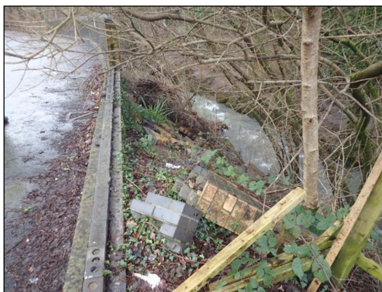
Figure 12: Damaged retaining wall at Melin Corrwg Business Park following the breach of the Nant Lonydd watercourse during Storm Dennis (image captured by RCT's Flood Risk Management team on 17 th February 2020)
