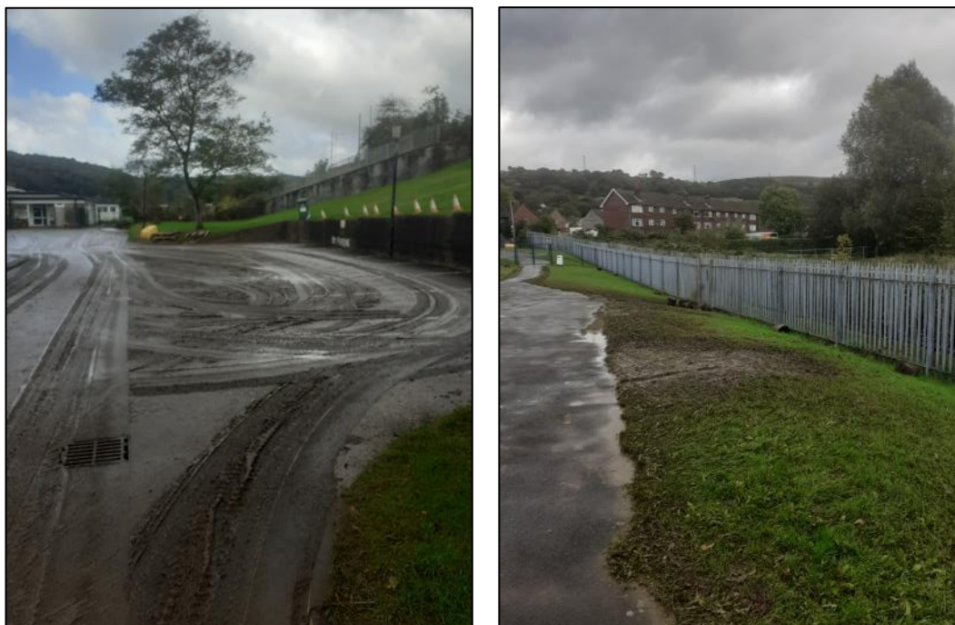
Figure 14: Mud and silt deposits (left) and evidence of saturated ground indicative of the flow path of water (right) within the grounds of Heol-y-Celyn School (captured by RCT's Flood Risk Management team on 5th October 2021)
