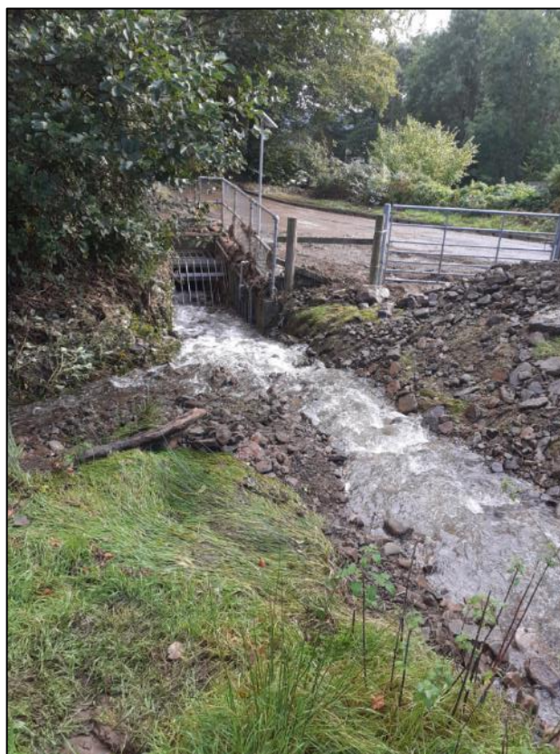
Figure 7: Image of 'Culvert Inlet RH03' showing material deposited on the channel banks during post event inspections (captured by RCT's Flood Risk Management team on 5 th October 2021)
