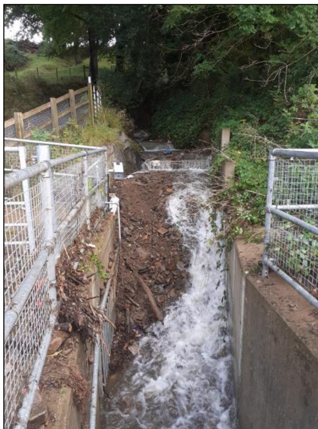
Figure 10: Image of 'Culvert Inlet RH02' showing material deposited within the channel during post event inspections (captured by RCT's Flood Risk Management team on 5 th October 2021)
