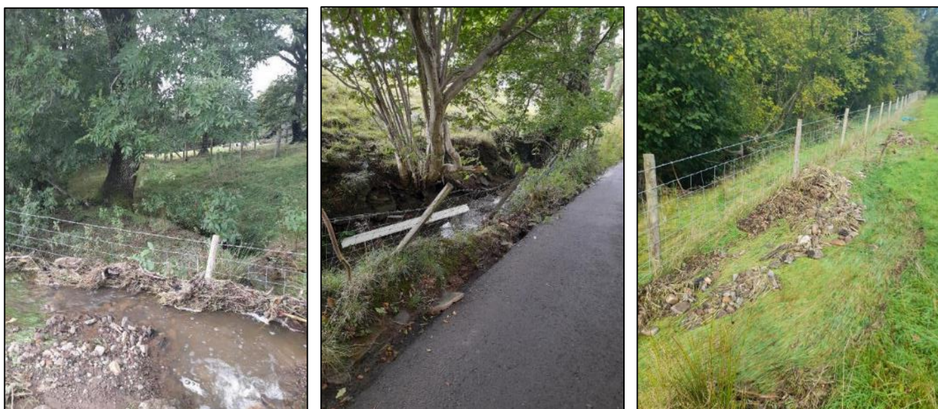
Figure 34: Obstruction of flow (left), scouring of the channel embankment and tarmac road (middle) and deposits of material indicative of out-of-bank flows (right) within RH02 Area 3 of 'Unnamed Ordinary Watercourse RH02' (images captured by RCT during post event inspections)
