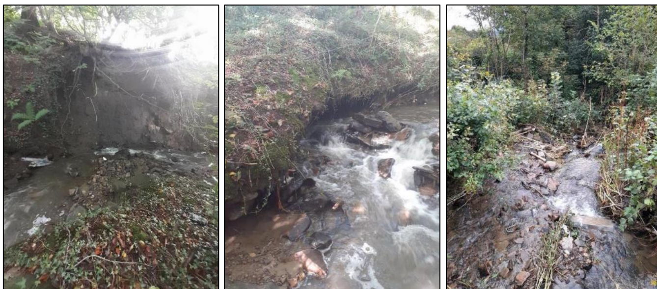
Figure 33: Evidence of significant embankment scour (left), undercutting (middle) and debris deposition (right) within RH02 Area 1 of 'Unnamed Ordinary Watercourse RH02' (images captured by RCT during post event inspections)
