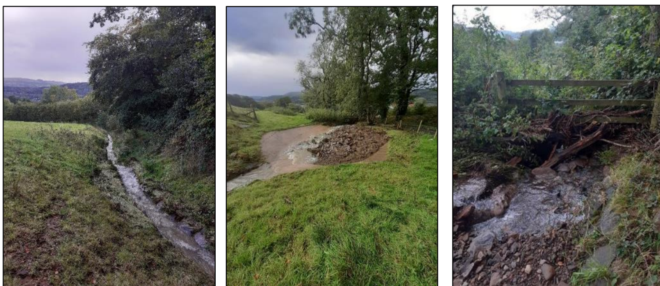
Figure 30: Evidence of the overtopping of 'Unnamed Ordinary Watercourse RH03' (left), debris accumulation at the ford (middle) and debris causing an impediment of flow (right) at RH03 Area 1 (images captured by RCT during post event inspections)
