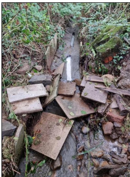
Figure 19: Obstruction of flow within the unnamed ordinary watercourse channel (captured by RCT's Flood Risk Management team on 8 th October 2021)
