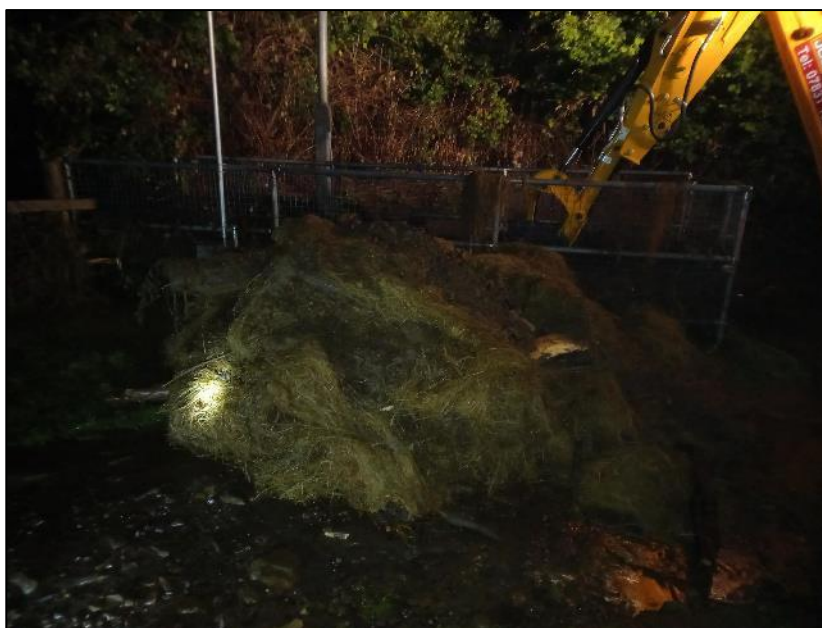
Figure 23: Image of the debris removed from 'Culvert Inlet RH03' during emergency clearance works carried out by RCT's Highway and Streetcare Depot on 5 th October 2021
