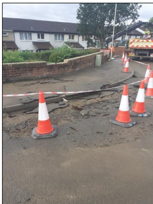
Figure 12: Damage to the highway at Wordsworth Gardens (captured by RCT's Flood Risk Management team on 5 th October 2021)
