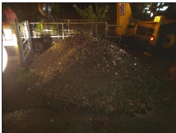
Figure 26: Image of the debris removed from 'Culvert Inlet RH02' during emergency clearance works carried out by RCT's Highway and Streetcare Depot on 5 th October 2021
