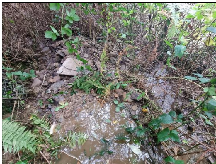
Figure 18: Silt and stone causing an impediment of flow within the unnamed ordinary watercourse channel (captured by RCT's Flood Risk Management team on 8 th October 2021)
