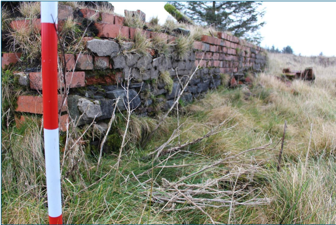
Plate 92. E facing view of Tramway Winding Engine House (TT04) showing detail of standing masonry fabric.
