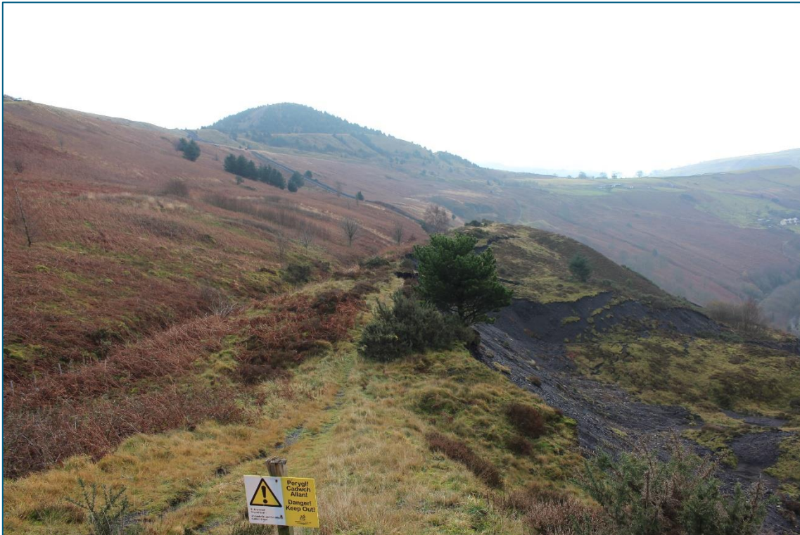
Plate 13. SE facing view of RH01 Tylorstown Upper Tip (TT01) looking towards the development area and showing damage caused by landslide. Tramway (TT03) can be seen in the centre distance.
