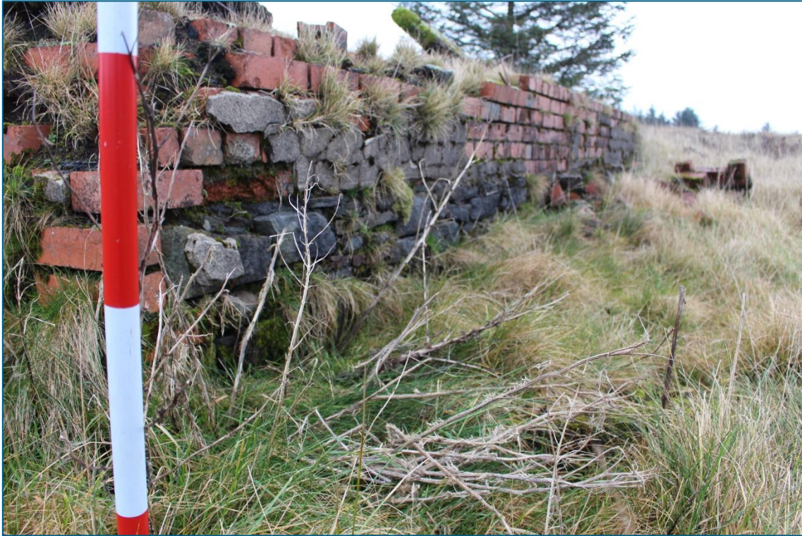
Plate 27. E facing view of Tramway Winding Engine House (TT04) showing detail of standing masonry fabric.
